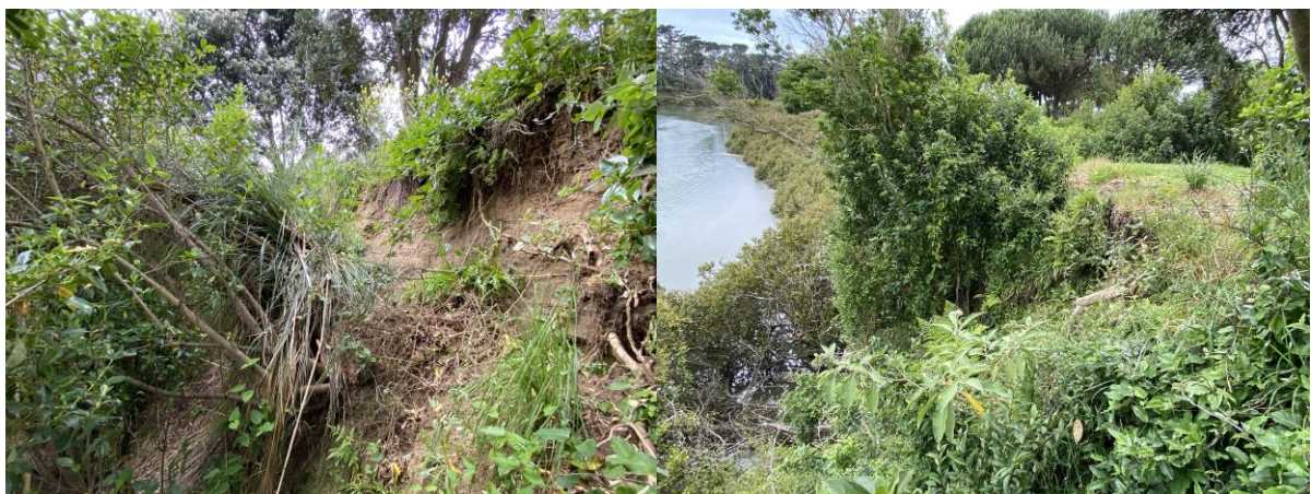
Figure 4: Slope instability due to bank erosion
