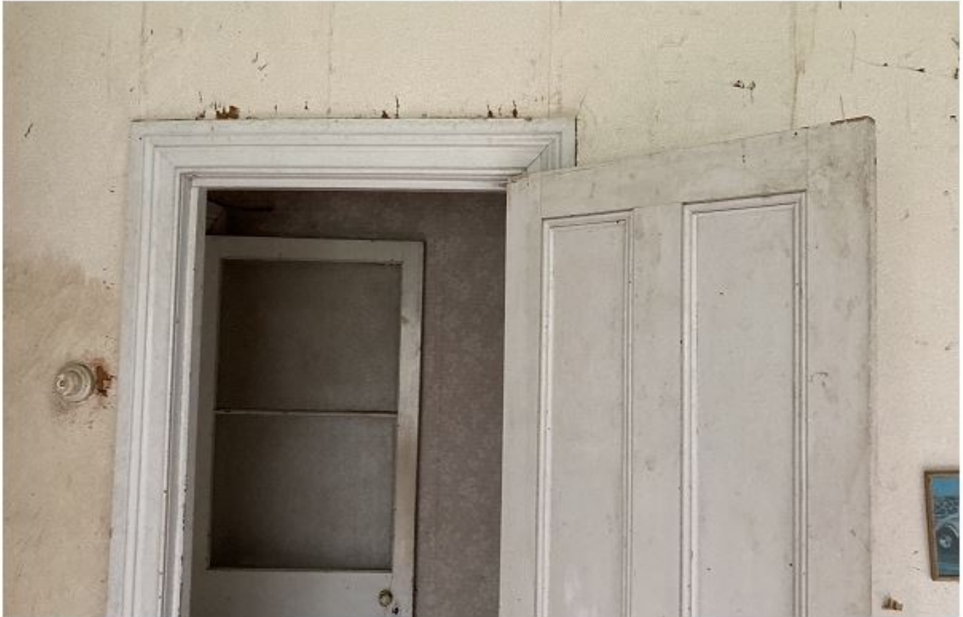
Original four-panel villa door and architraves. Beyond is the hall door minus original glazing and all but one glazing bar.
