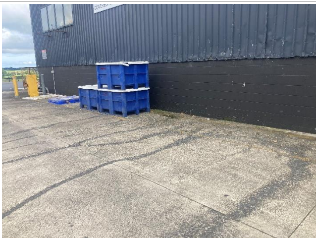
Photo 3: Etching in concrete from waste storage area, draining down to a stormwater sump.
