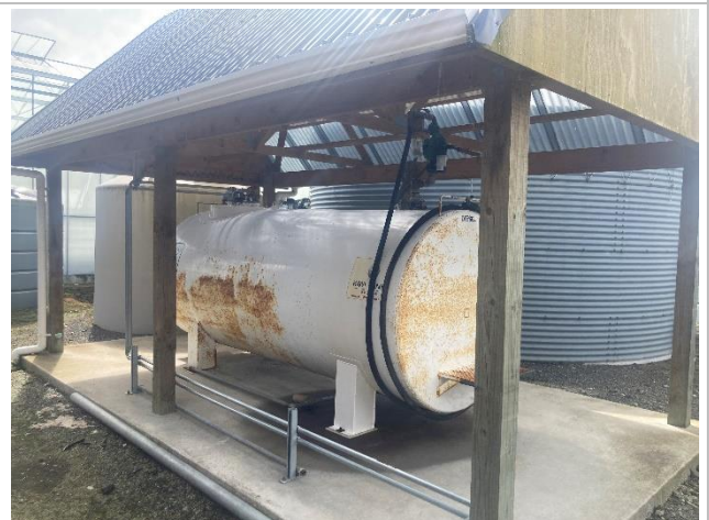
Photo 25: Old AST in water tank compound, currently being decommissioned.
