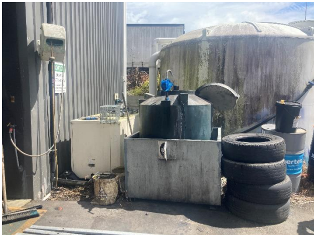
Photo 13: Waste oil storage, transformer and water tanks external to the workshop
