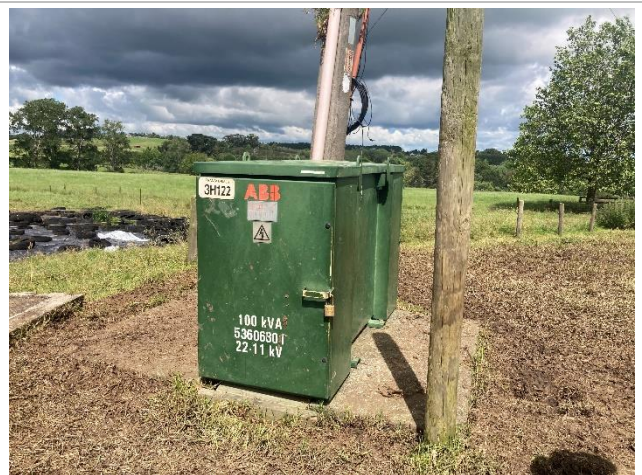
Photo 35: Transformer at 370 Karaka Road
