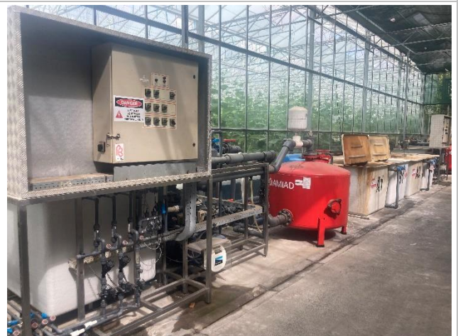
Photo 19: Automatic fertiliser dosing system. The mixing bins are in the rear of the photo and floor drain is visible.
