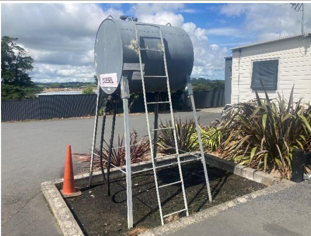
Photo 9: Diesel tank. Hydrocarbon staining below.
