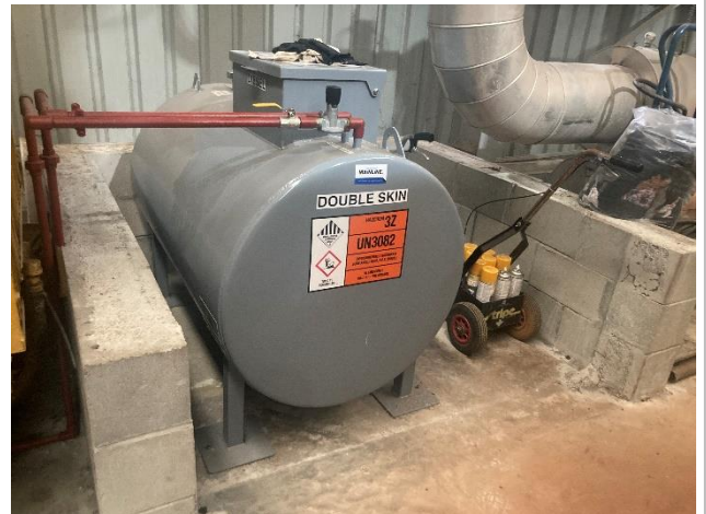
Photo 23: Diesel storage within the boiler room
