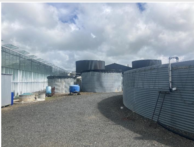
Photo 24: Water tanks – cold water tanks in the foreground and the tall hot-water tanks in the background.
