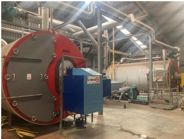
Photo 22: The two boilers, one for each half of the glasshouses
