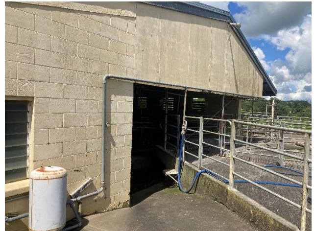
Photo 37: Likely ACM cladding on the northern apex. Concrete block is also visible.
