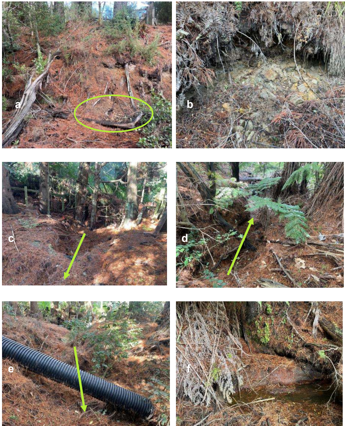
Figure 7: Site observations of the coastal edge at 16 Sinton Road. Observations of bank slumping (see green circle in photo a) undercutting and erosion of the bank toe (b), OLFP (c, d with arrow showing likely direction of flow), nova coil pipe that sits above the OLFP (e, arrow showing direction of flow of OLFP) and exposed sandstone and pool in CMA (f).
