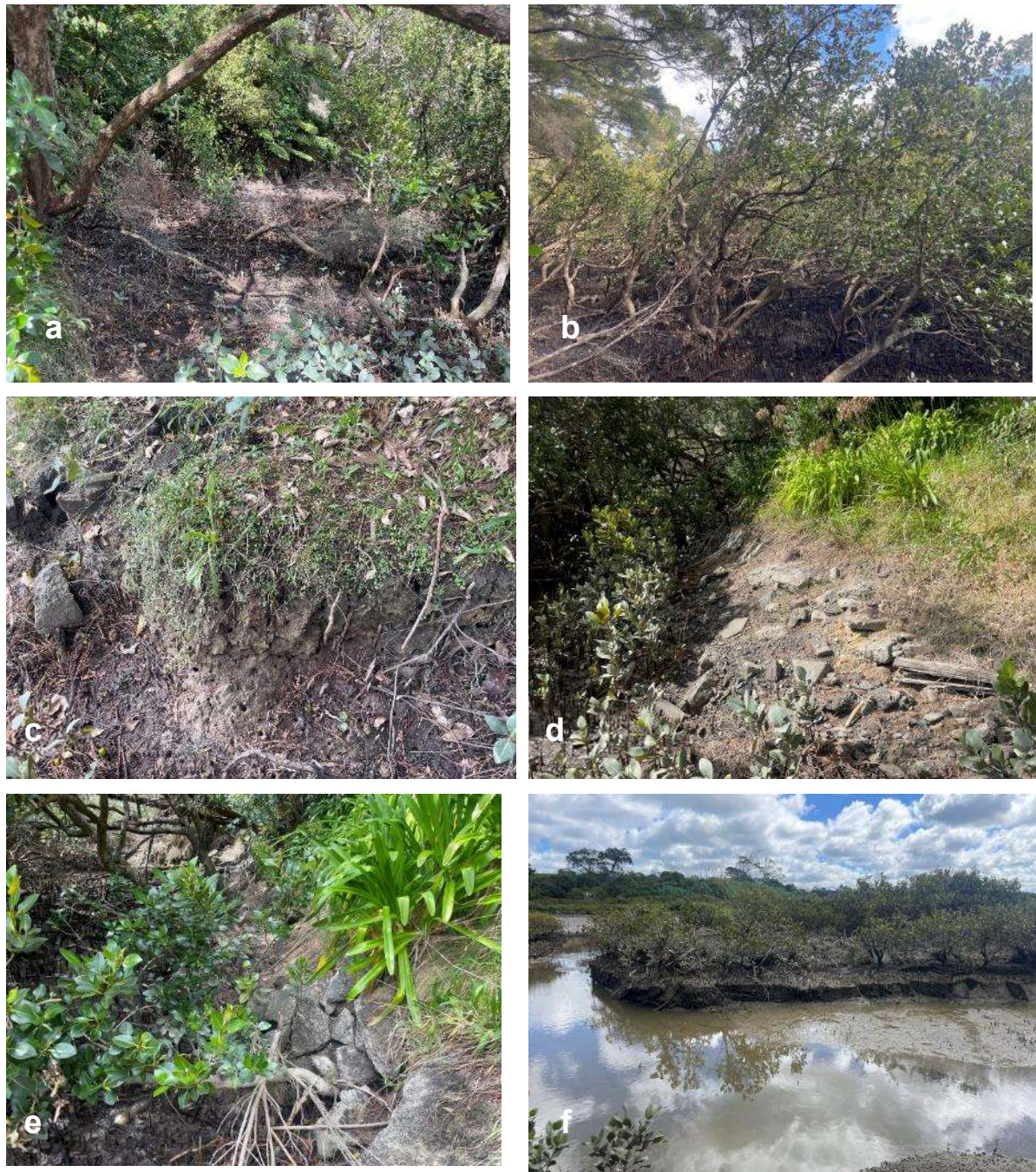
Figure 6: Site observations of the vegetated bank looking west towards the Significant Ecological Area (a, SEA_T_4733), fronted by mangroves and tidal flats (b), section of the bank toe with mud crab holes and cracks (c), riprap and concrete of an informal seawall (d, e) and evidence of dug sections of the mudflat by machinery for boating access (e).
